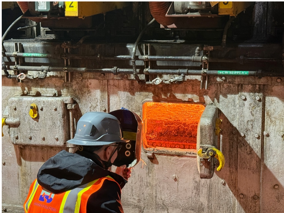
Figure 6: Workshop participant observes the feed mechanism and combustion chamber of a coal boiler during a tour of the Fort Wainwright Combined Heat and Power Plant.
