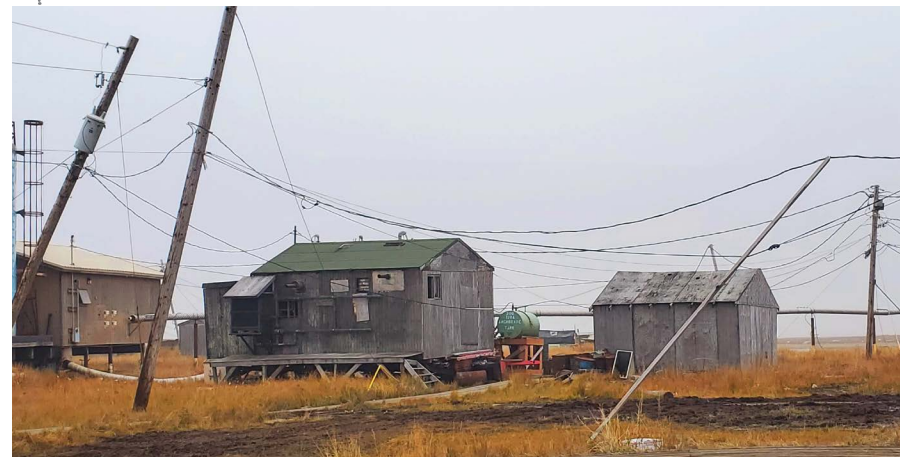
Power poles in Newtok, Alaska. Image credit: Alaska Native Tribal Health Consortium
