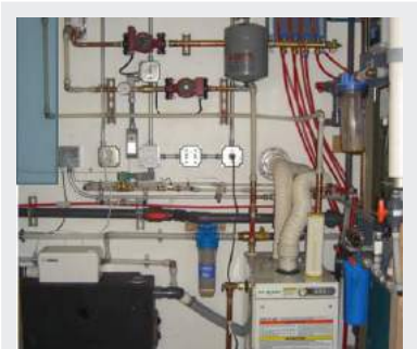
Waste water storage tank, drinking water filters and freeze-thaw protection using heat trace pipes
