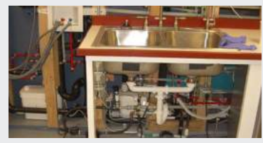
Wash water and drinking water are available at the kitchen sink.
